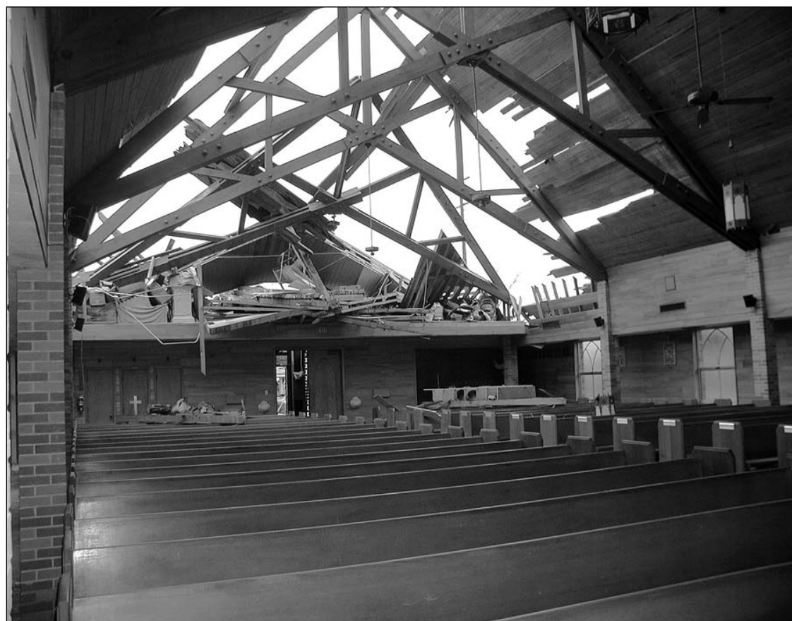
A major portion of the roof of St. Peter the Apostle Church in Hackberry Parish was ripped off allowing rain to flood the church. The Church hall and the rectory also received major damage.
