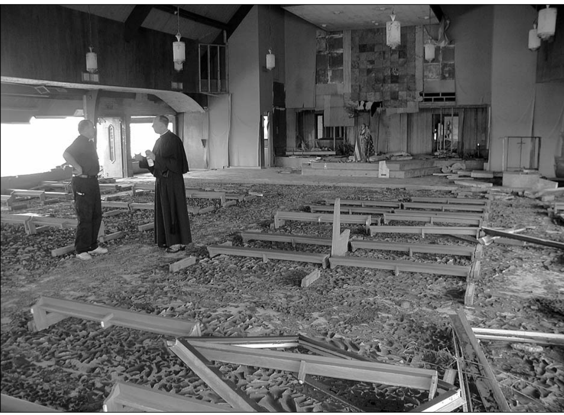
Fr. Joseph McGrath, right, and Msgr. Harry D. Greig, left, talk about the damage to Sacred Heart of Jesus Church in Creole. Every pew in the church was gone but almost all of the kneelers remained. Fr. McGrath's house and the church hall were also devastated.
