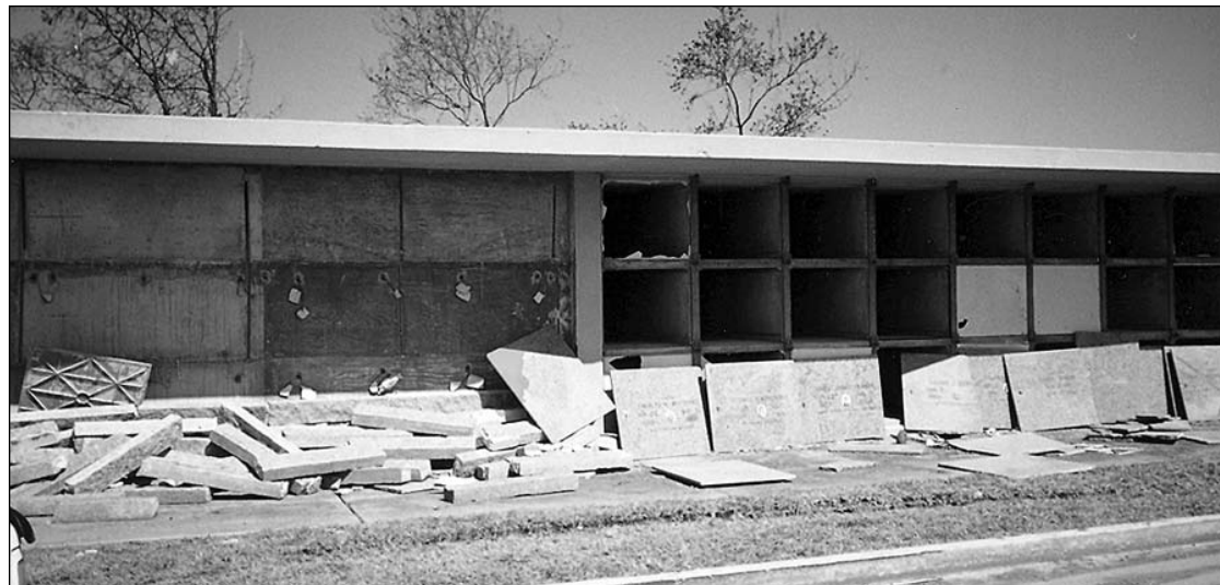
Damage was severe due to Hurricane Rita at the mausoleums of Sacred Heart of Jesus Church in Creole and Our Lady Star of the Sea Church in Cameron. Broken pieces of granite as well as whole doors that may be reusable are shown here at Sacred Heart. Work will begin soon to repair the facilities.
