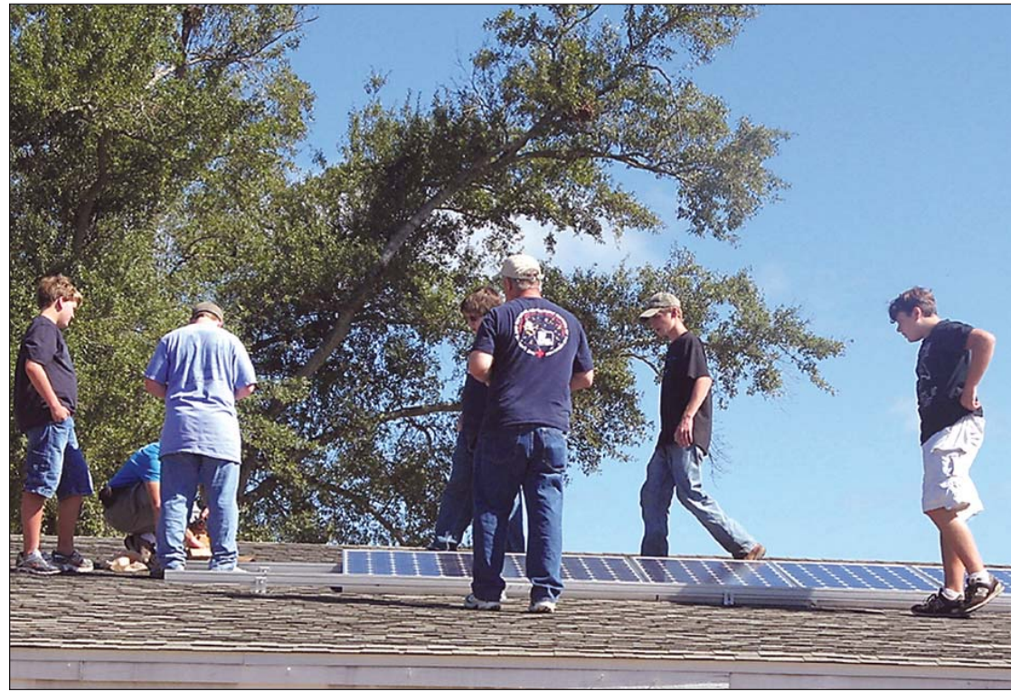
Members of the St. Margaret of Scotland Catholic School help with the installation of solar panels. The project was the brainchild of St. Margaret graduate Thomas Breaux who came up with the idea as part of the process of earning his Eagle Scout award. The school is the first in the State of Louisiana to have solar power. The panels produce twice as much electricity as that needed to operate the school's science classroom and science lab.
